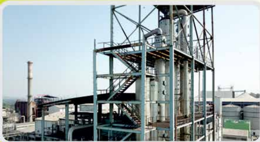
500 KLPD Grain Based Ethanol Plant at Boregaon, Madhya Pradesh
